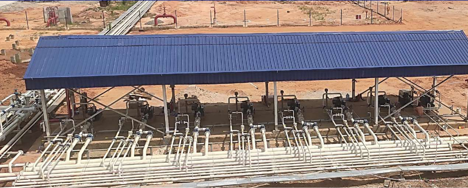
PROCESS PUMP HOUSE
